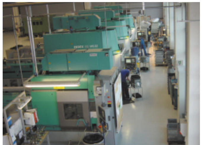
Easy access: The switch cabinet was relocated horizontally on the top of the machine
